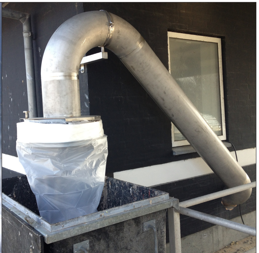
Outside pipe for pressed screen solids.
