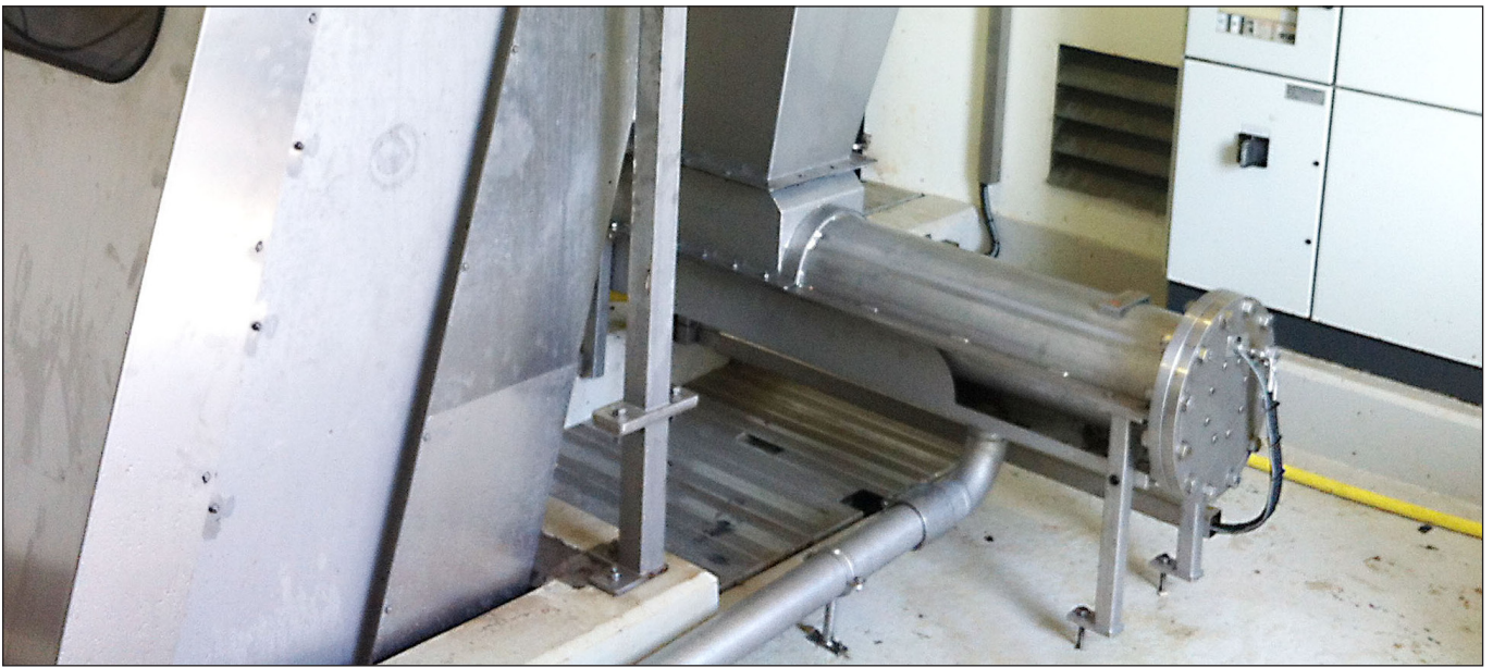
Kerteminde WWTP, Denmark.
