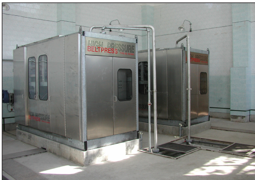
2 x KD 10-1500 - Brest WWTP
