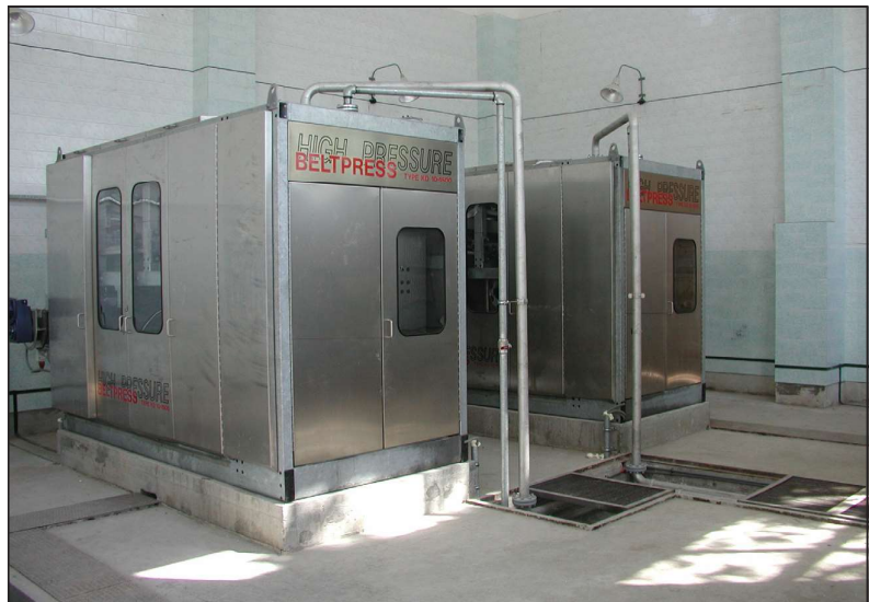
2 x KD 10-1500 - Brest WWTP
